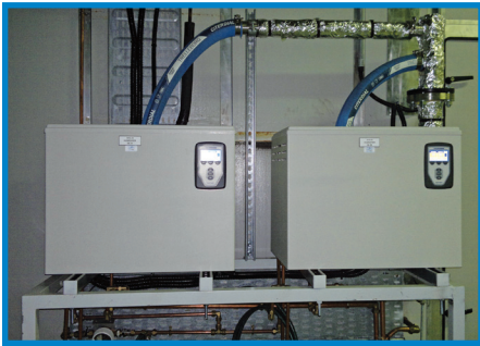
Installed Vapormist humidifiers at BSCL.
