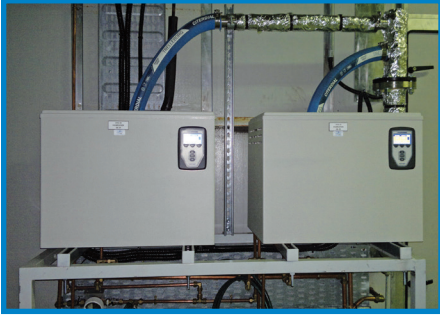
Installed Vapormist humidifiers at BSCL.
