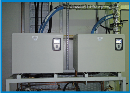
Installed Humidi-tech humidifiers at BSCL.
