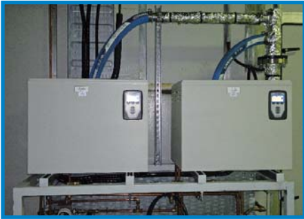
Installed Humidi-tech humidifiers at BSCL.
