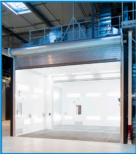
Aircraft paint booth. Bright, clean, and perfectly humidified and ventilated by DriSteem and Sima.
