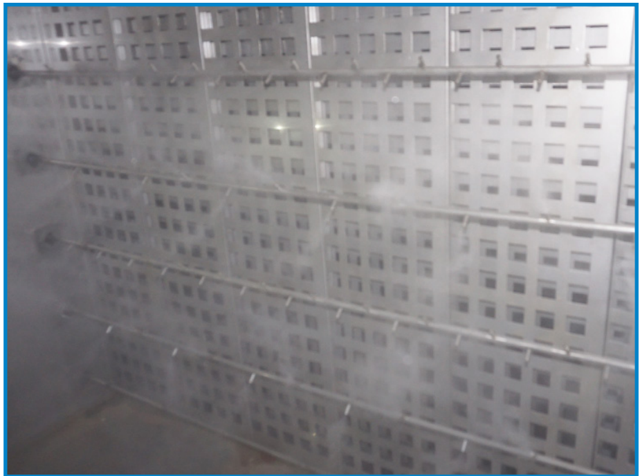
High-pressure system atomizing nozzles disperse ultra-fine water droplets into five air handlers. Four air handlers move 40 000 cubic meters/hr of air; the fifth air handler moves 28 000 cubic meters/hr.
