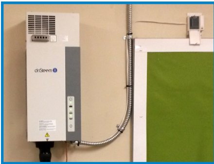
DriSteed XTR electrode steam humidifier in one of the two humidified classrooms at the Aldrich Memorial Nursery School
