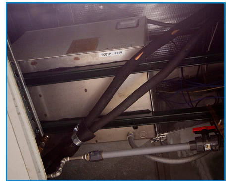
Vapormist ® electric humidifier installed above a busy hallway. Two ducts bring steam from this unit into the data center.
