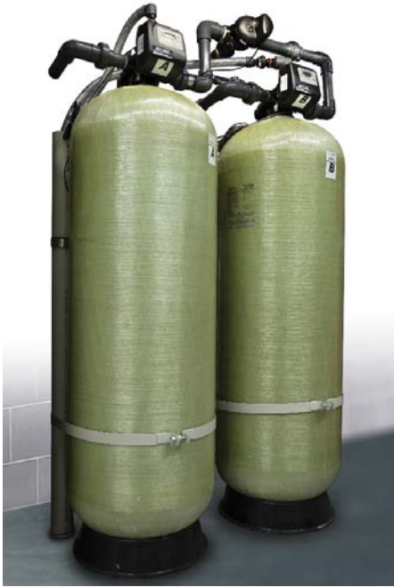
FIGURE 4-1: DUPLEX WATER SOFTENER AND BRINE TANK
